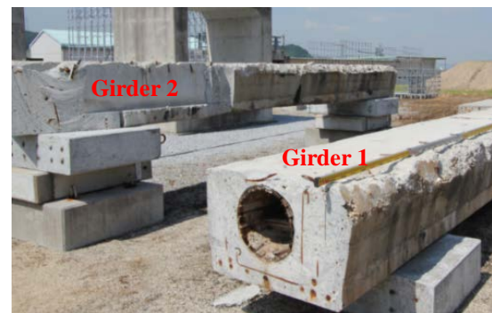
Fig.5 PC digit removed due to salt damage
