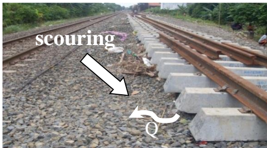
Fig.1. The scouring of rail ballast after flooding
