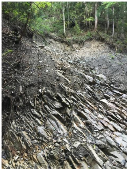
Fig.6 Bedrock layer of the landslide scar
