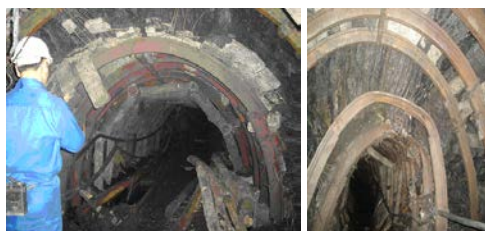
Fig. 1 Failure mode of passive support in Trang bach coal mine
