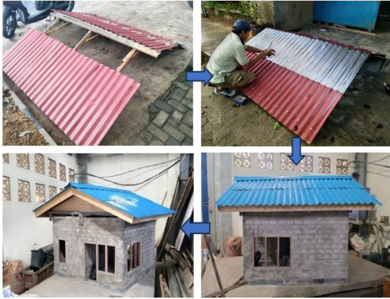
Fig.10 Fabrication of the roof frame and installation of the roof on the specimen
